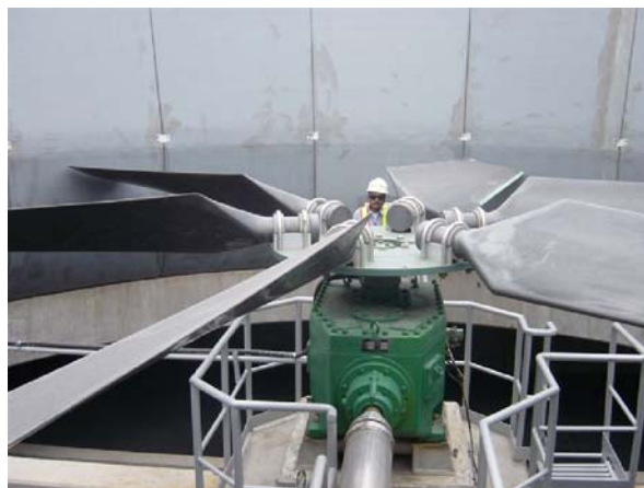
Figure 3. Installed air cooled fan
