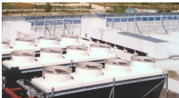
Figure 1. Air cooled condenser bank
