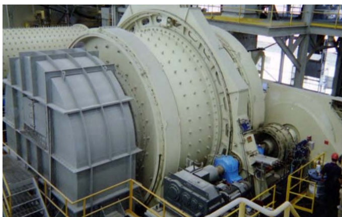
Figure 2. Grinding mill installation
