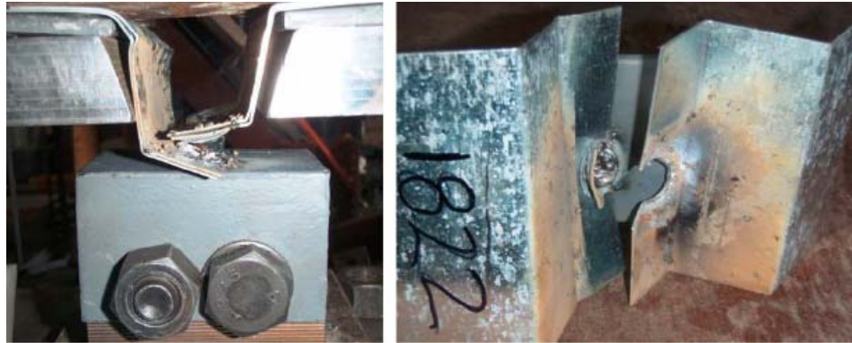
Figure 1.7: Tension sheet failure (Guenfoud, 2010).
