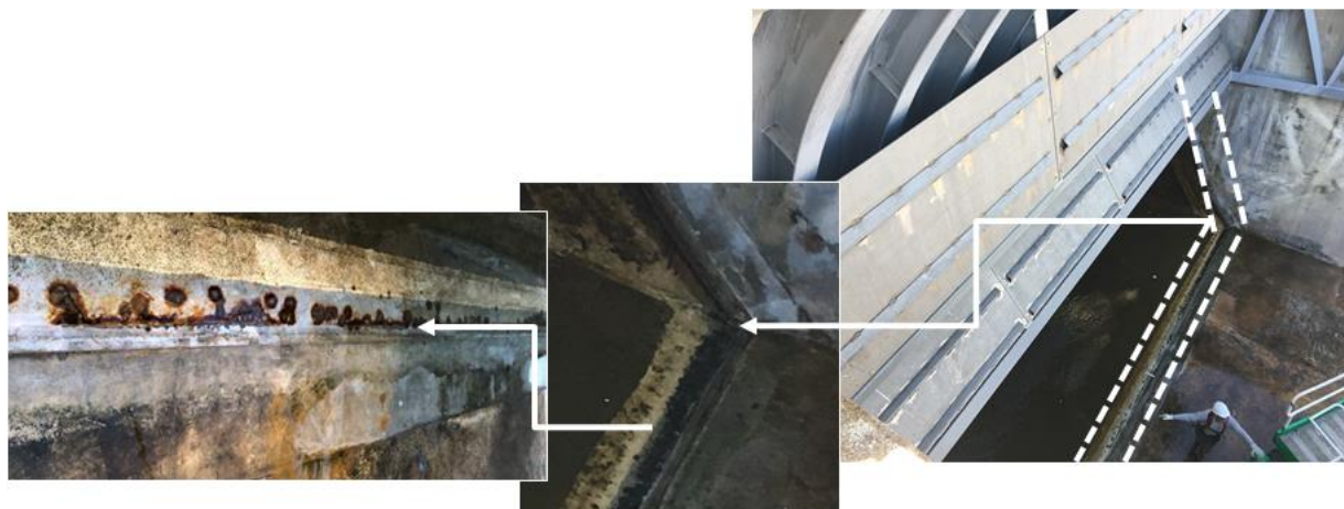
Figure 3: Corrosion Morphology and Location for the Stainless Steel Embedment Plate
