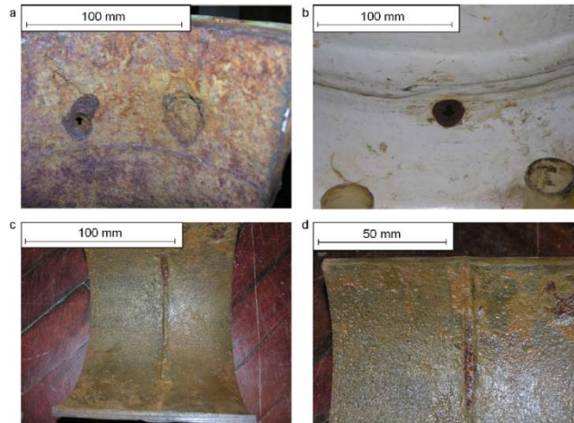
Figure 2: Erosion-corrosion degradation (Xinming Hu, Richard Barker, Case study on erosion–corrosion degradation of pipework located on an offshore oil and gas facility)
