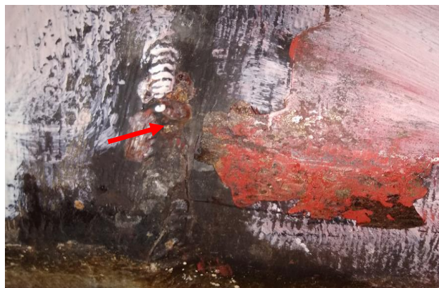
Photograph No. 6 – Location #1, Spot Rust on Pipe Cable
