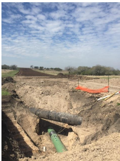
Figure 2: Newly constructed pipe with sensors installed at the low spot of the pipeline segment
