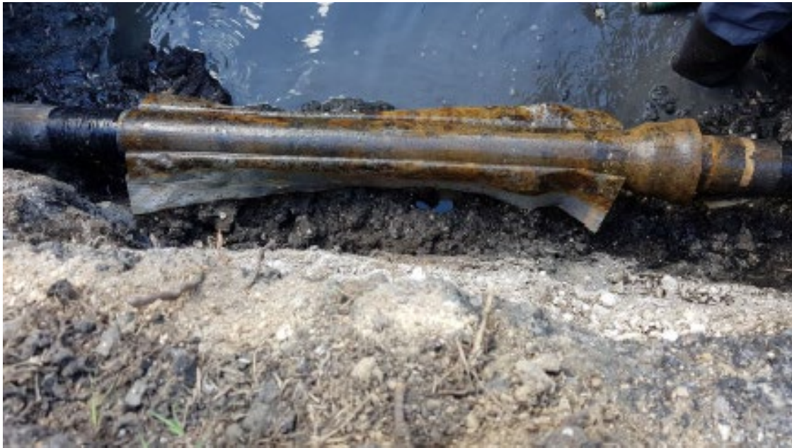
Figure 3: The film was removed from the pipe prior to shipment to laboratory for physical testing. Oxidation is visible on the surface of the pipe prior to cleaning.
