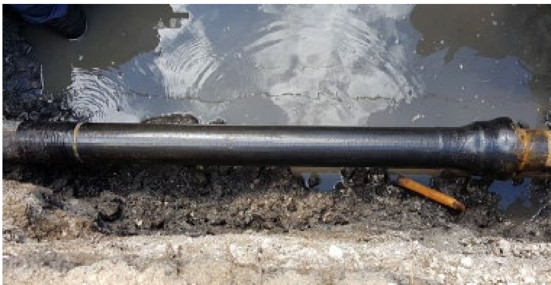
Figure 4: The surface of the exposed pipe has been cleaned using a wire brush and water. The oxidation was removed and found to be superficial.
