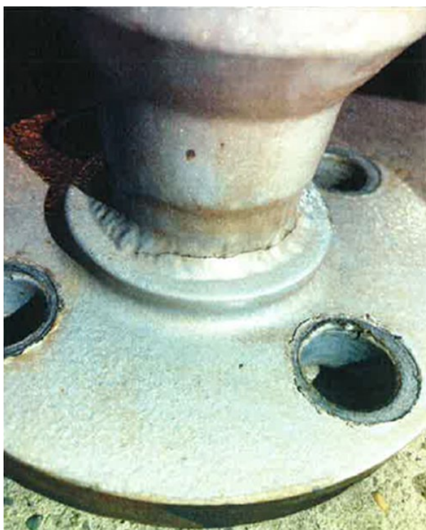
Figure 1: Socket weld failure and crack
