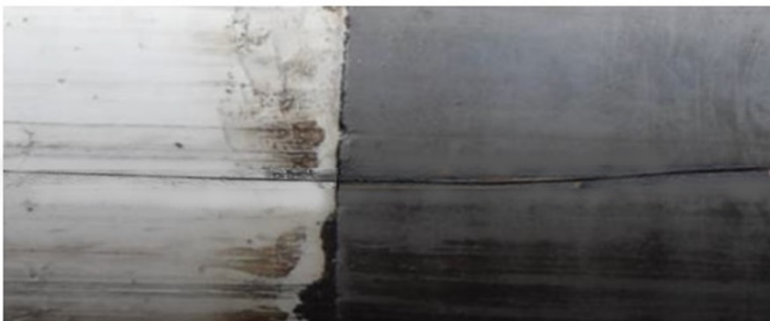
Figure 2: Propagated crack due to release of internal stresses on a 3LPP coated pipe
