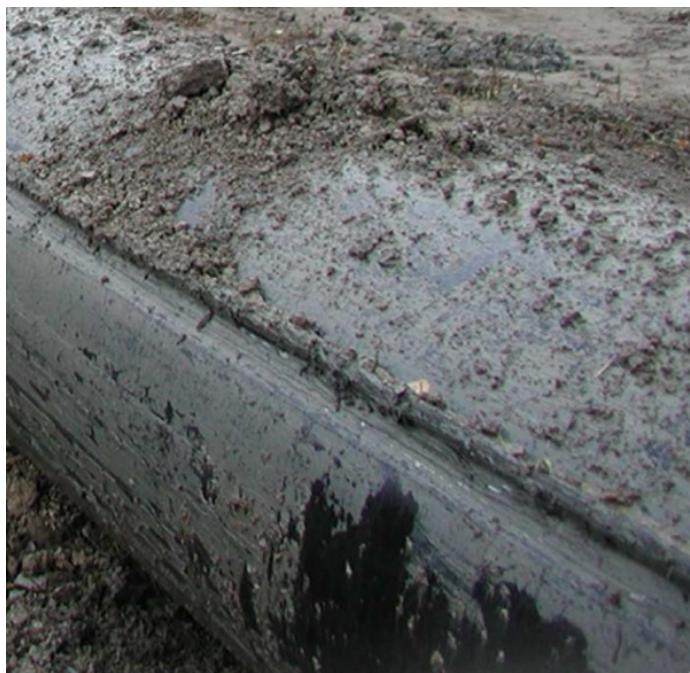
Figure 1: Deep scratch damage during an HDD project
