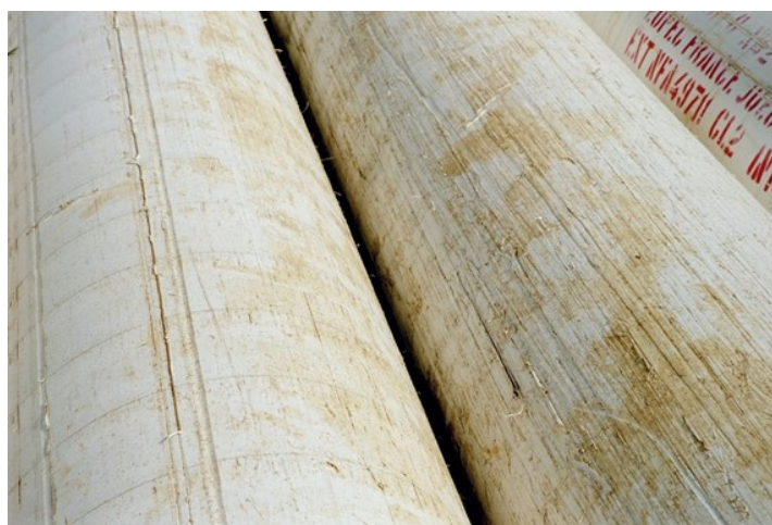
Figure 3: Deep scratches occurred due to gouging of polypropylene coating
