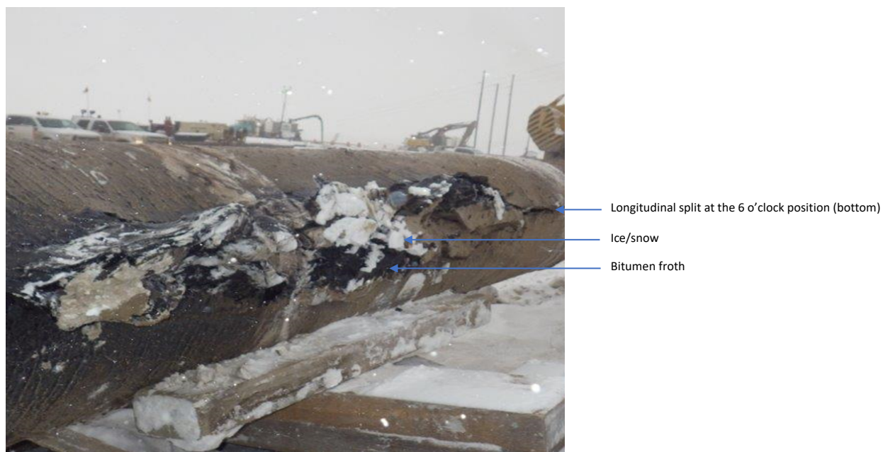
Figure 2: Failed spool after removal from the pipeline, showing the split at the 6 o'clock position propagated on a fairly straight manner over 12 m in length.
