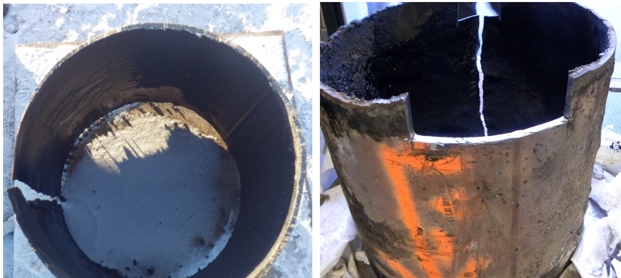
Figure 5: Pipe section cut out of the failed spool for further analysis.
