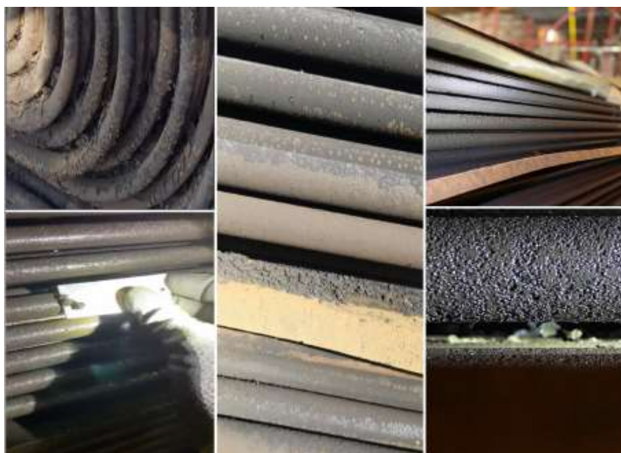
Figure 3: Solid deposits at reboilers of the NGLF De-ethanizer unit.
