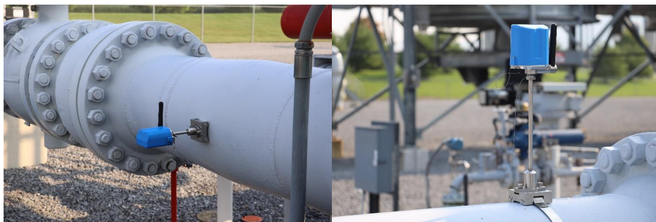
Figure 1: Wireless UT Sensors Installed on Refinery Assets
