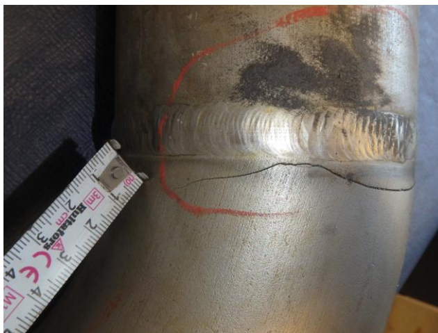
Figure 1: Overview of elbow with crack
