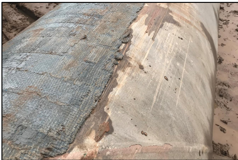
Figure 1: Photograph of representative coating damage during an HDD.
