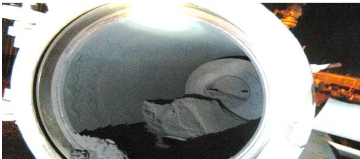
Figure 1: Black Powder Accumulation in Fuel Gas Pipeline FG-098
