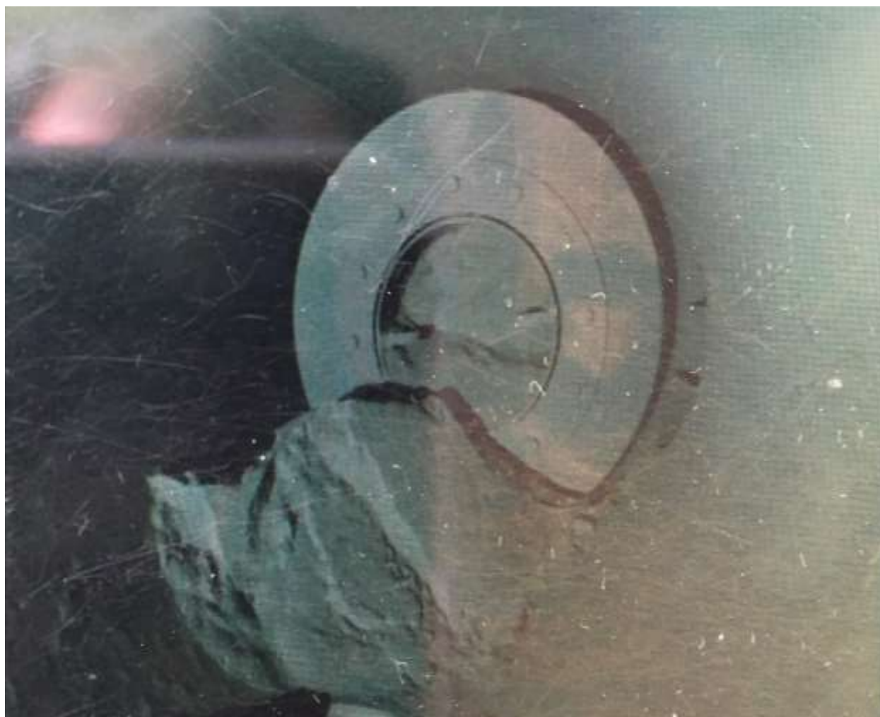
Figure 2: Black Powder Accumulation in Fuel Gas Pipeline FG-098
