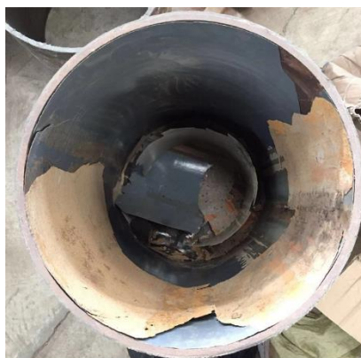
Figure 1: Corrosion morphology of field of the failure tubing
