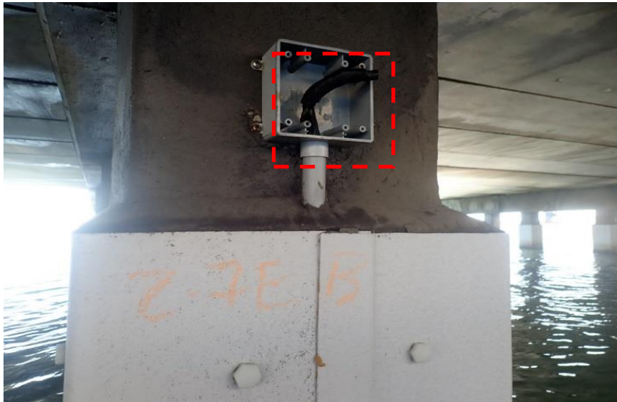
Figure 4: Heat shrink sleeve over electrical connections
