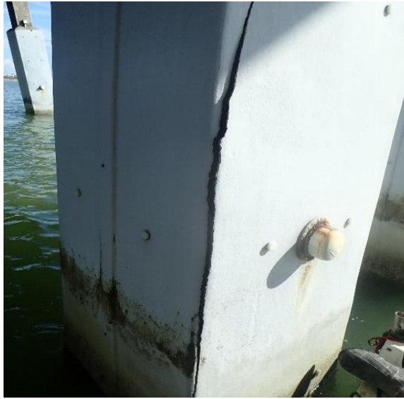
Figure 2: Large vertical crack exposing grout to environment
