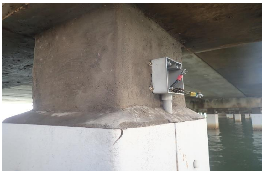
Figure 1: Typical small cracks at jacket corners
