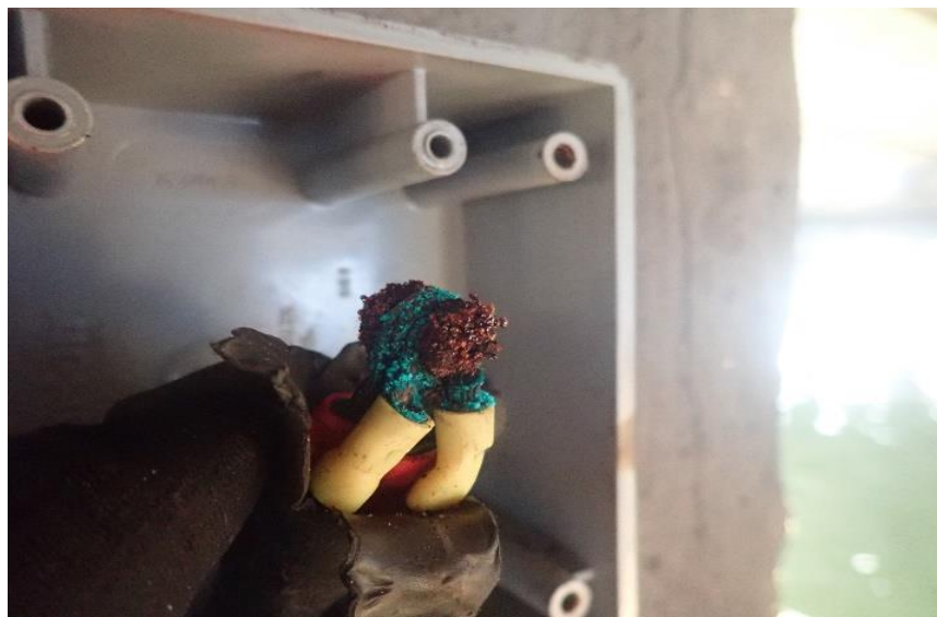
Figure 5: Corroded electrical connections inside junction box
