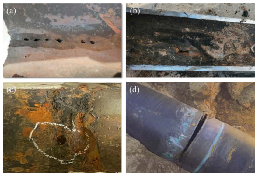
Figure 1: Typical morphologies of corrosion induced failure of ground gathering pipelines
