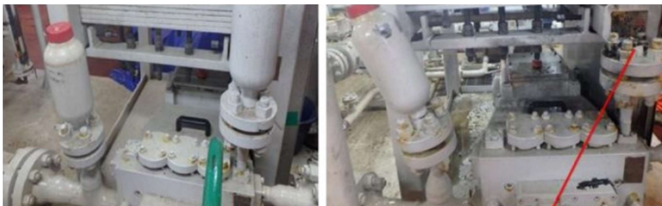
Figure 2: Location of dampener on site
