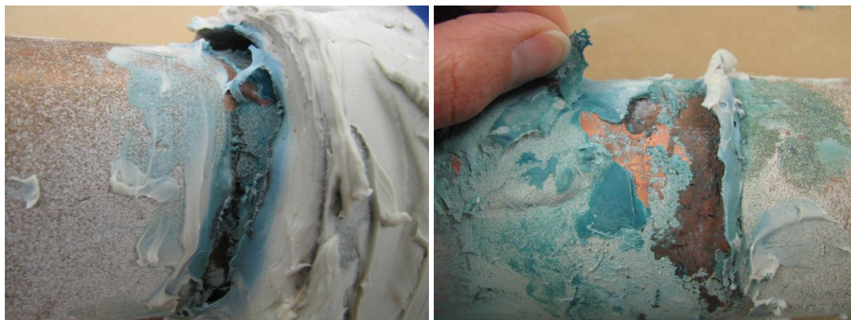
Figure 3: Sample A, showing discoloration of sealant and copper at contact location (left) and shiny copper when sealant was removed (right).
