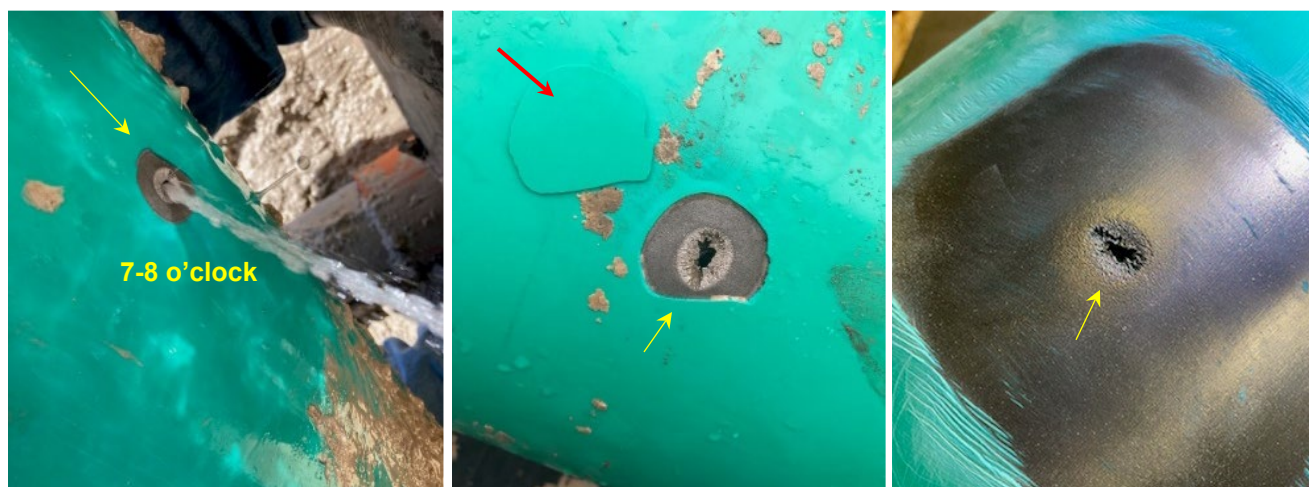
Figure 1. Photographs showing the leak during hydrostatic testing.
