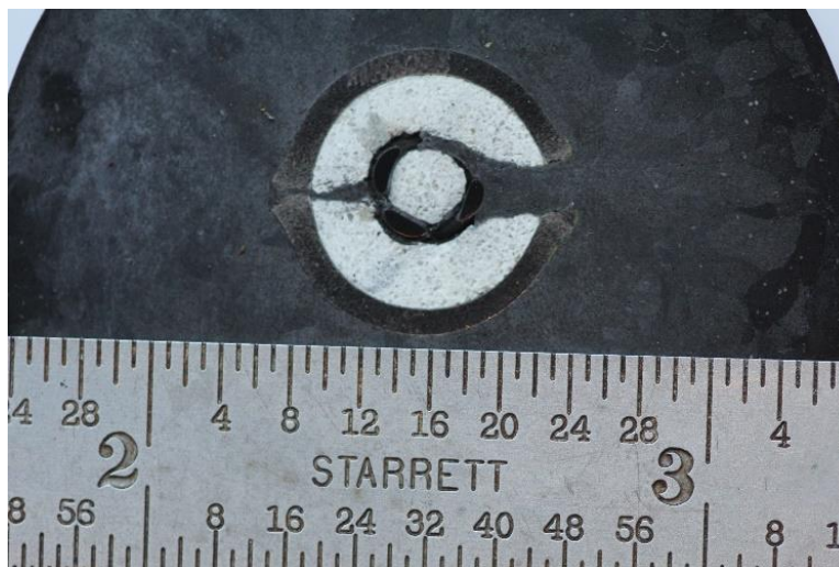
Figure 4: A cross-section view of tube #1 showing both extrados (right) and intrados cracks (left) of the hairpin bend portion.
