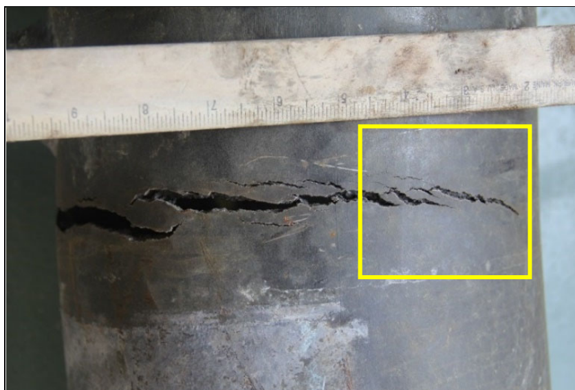
Figure 3: Close-up image of the crack.
