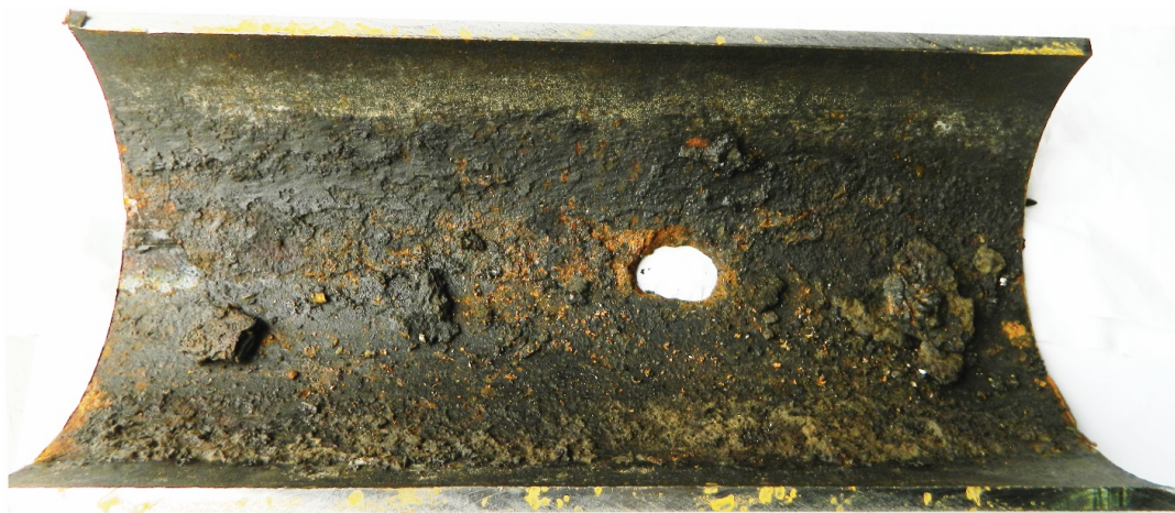
Figure 1: Brown-orange deposit near perforation and thick black loose deposits away from perforation (5 to 7 o'clock) observed on FL1. SRB's were detected in the black deposit
