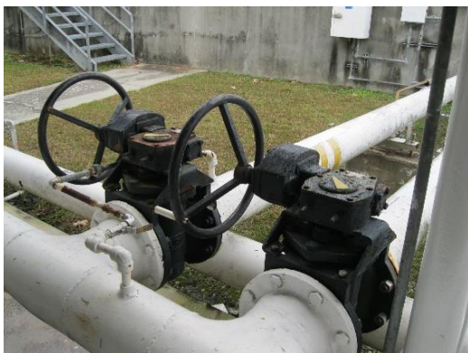
Photo 1. Various items are inventoried: valves, valve handles, and pipelines.
