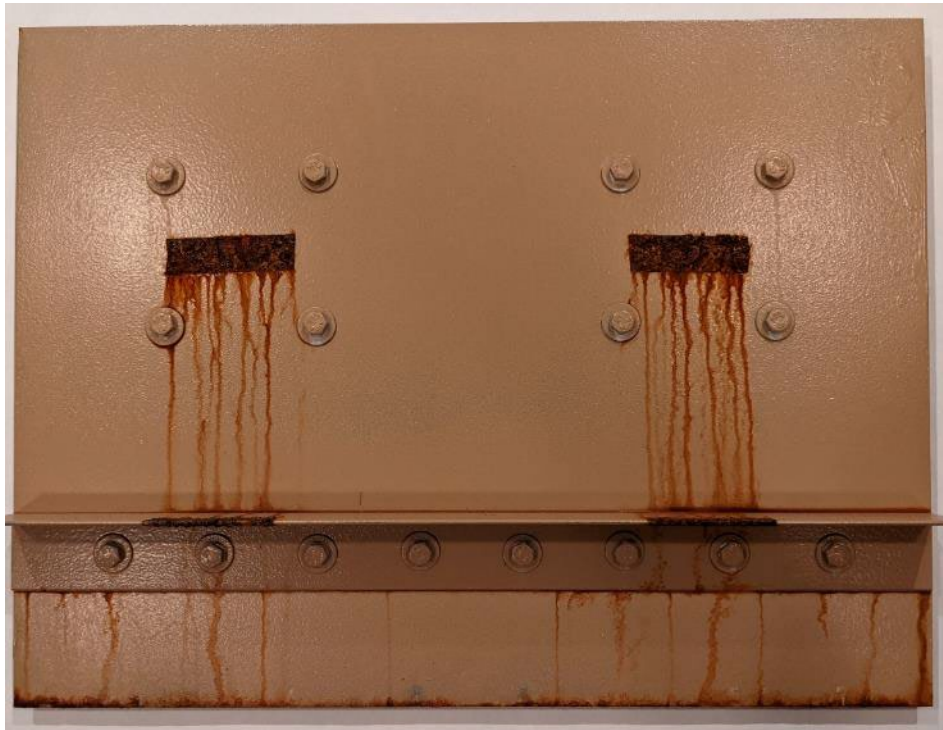
Figure 2. Large 18"x18" after Weathering
