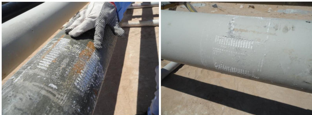
Figure 4: Coating Damage observed in gripped pipe
