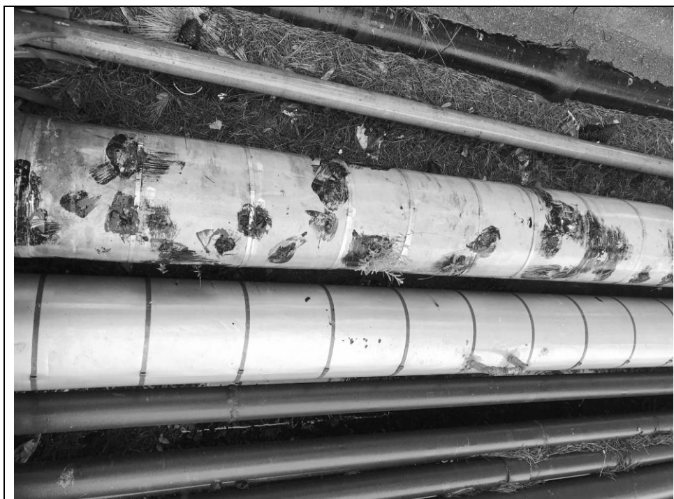
Figure 1; Patch Repairs and plant growth
