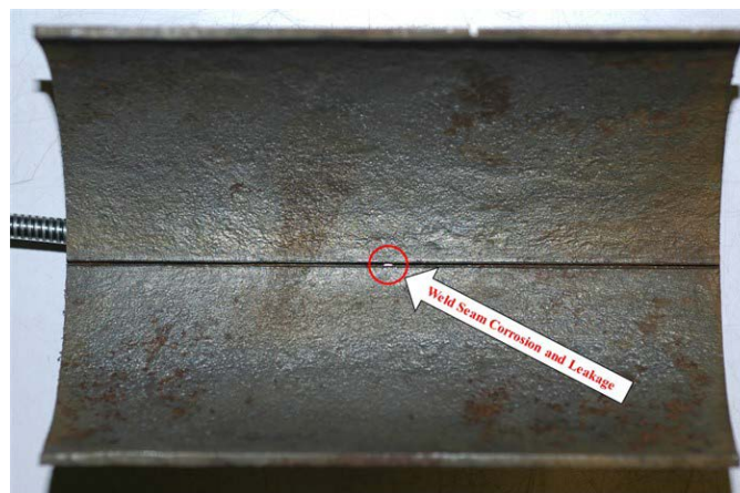
Figure 3: Photograph Showing Preferential Grooving Corrosion on Pipe Weld Seam with a 1 mm Pinhole Leak in a Wet Pipe System, after Removing Corrosion Products inside an NPS 3 Pipe (Image Courtesy of FM Global. Used with Permission. © 2014 FM Global. All Rights Reserved).
