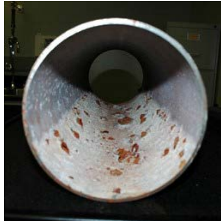
Figure 1: Photograph Showing Corrosion of Galvanized Steel Pipe (NPS 6, Schedule 10) Where Residual Water Filled Approximately 40% of the Pipe's Volume in a Dry Pipe System (Image Courtesy of FM Global. Used with Permission. © 2014 FM Global. All Rights Reserved).
