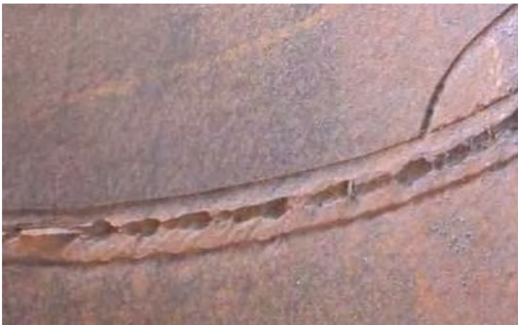
Figure 3-2-3—Preferential weld corrosion in lean amine. (Reference 5)
