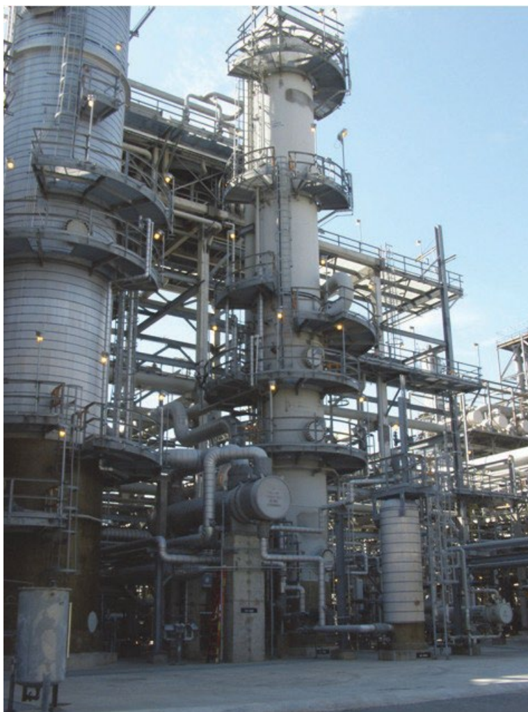
Figure 1—Example of a Process Tower
