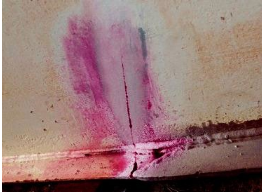
Figure 16—Cracks in Tank Shell Plate
