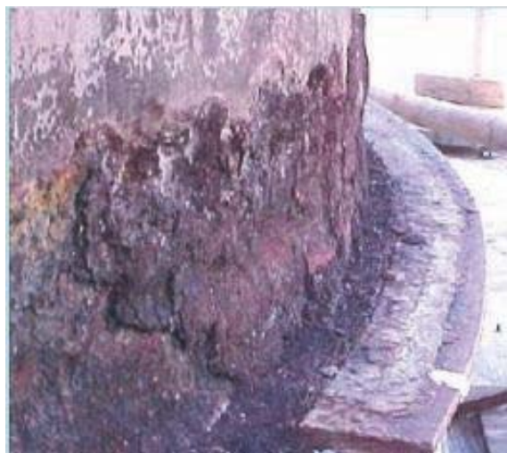
Figure 4—CUI at an Insulation Support Ring
