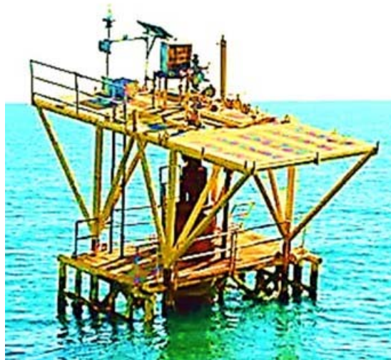
Figure 3.1—Example Caisson Platform Leaning Damage
