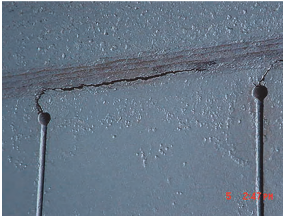
Figure 7—Keyhole Skirt-to-Bottom Head Weld Cracks
