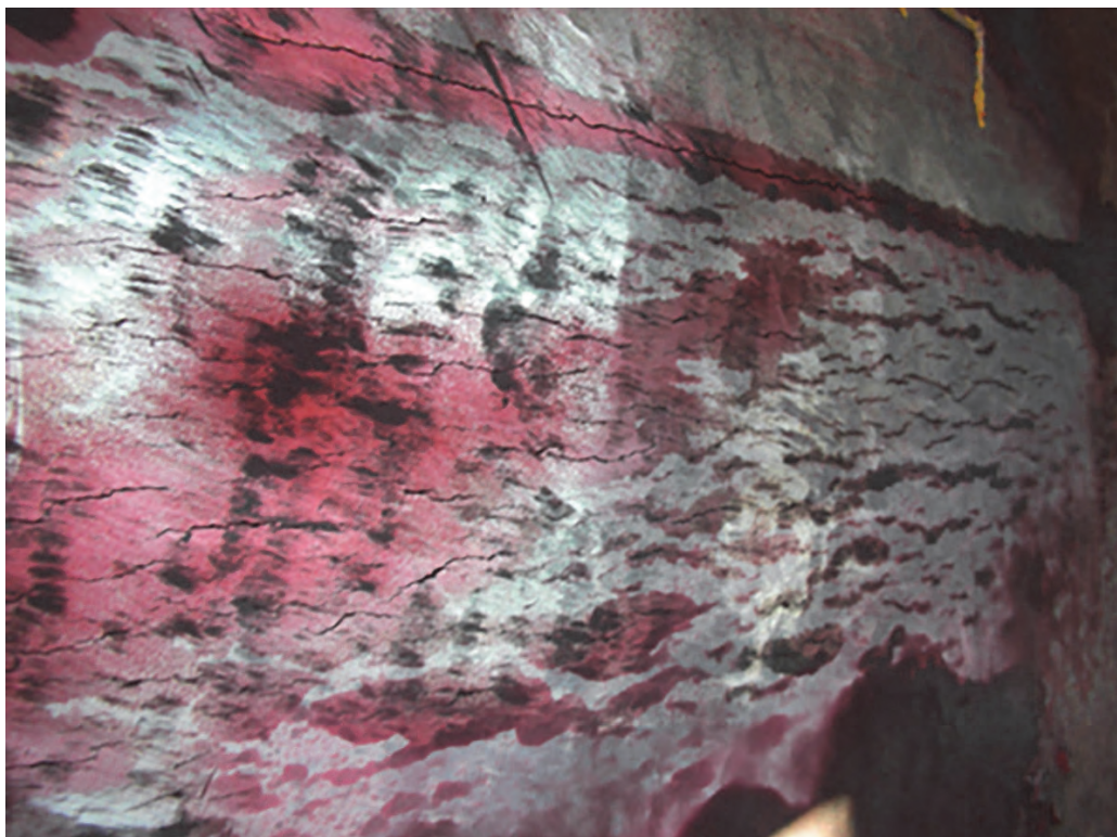
Figure 9b—External Surface Bulge Cracks
