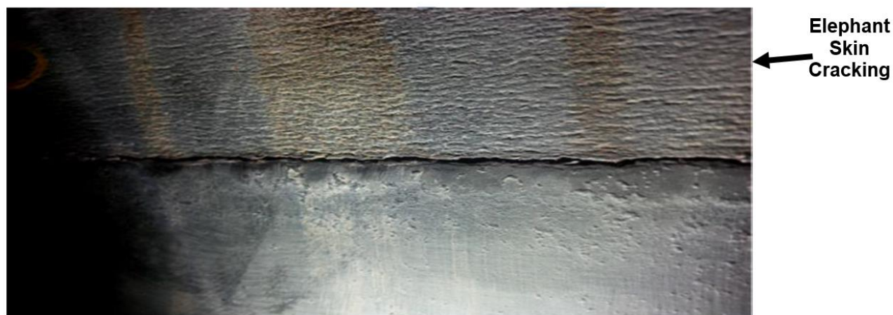
Figure 1—VT Examination of a Coke Drum Surface That Displays “Elephant Skin” Cracking
