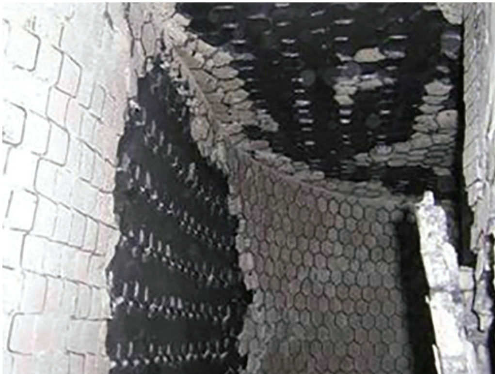
Figure 4—Large Areas of Internal Hexagonal Mesh and Refractory that Failed in a Brittle Manner
