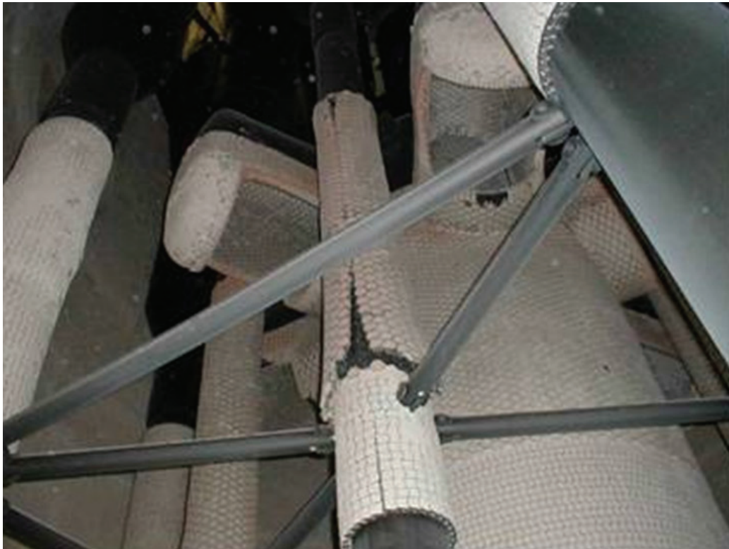
Figure 5—Example of External Refractory that Failed After a Short Time in Service
