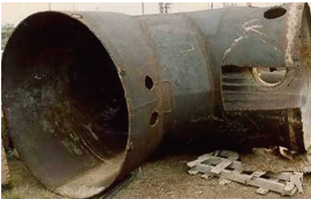
Figure 6—An Example of a Mitered Joint After Removal From Service
