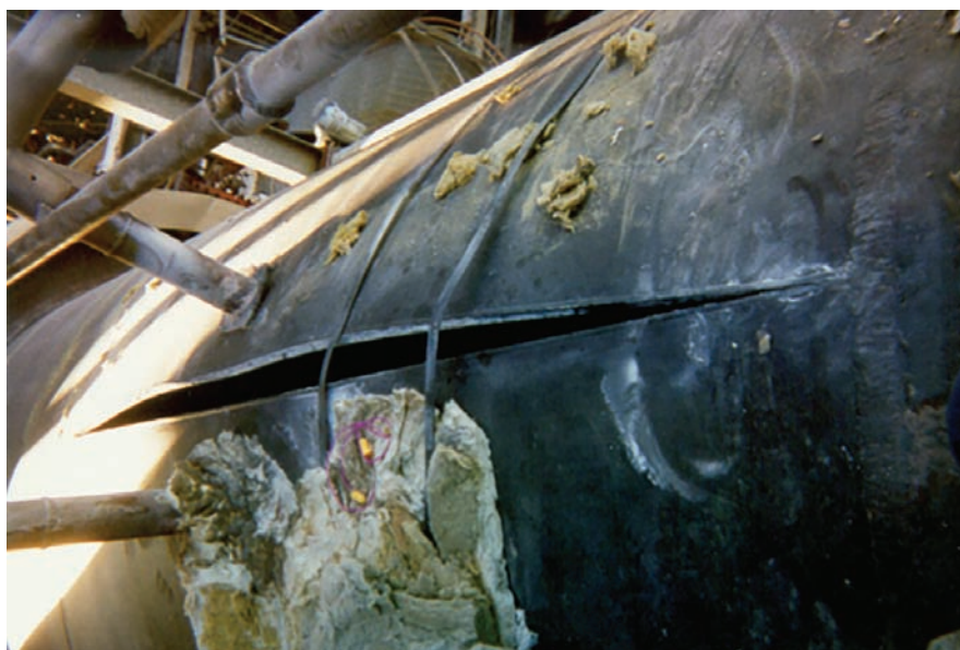
Figure 7—Creep Failure on a FCCU Regenerator Overhead Line
