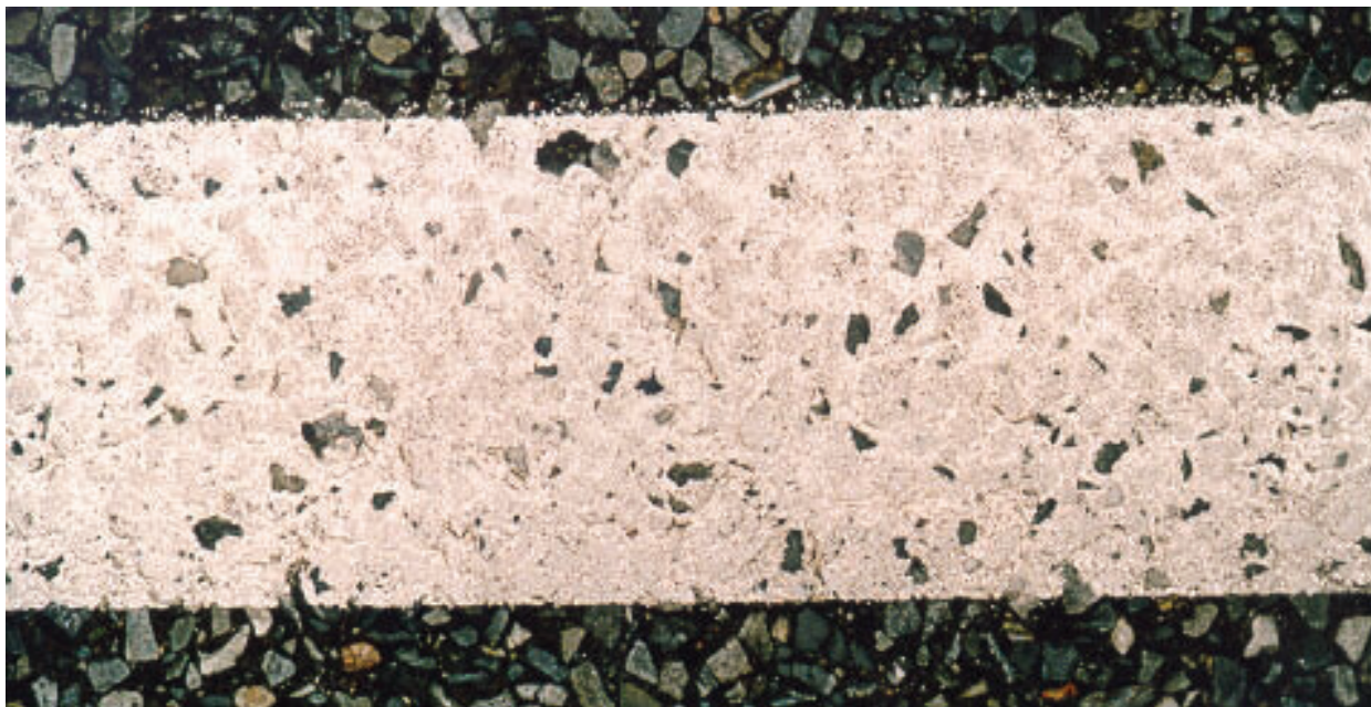
FIGURE L2 90% OF AREA INTACT
