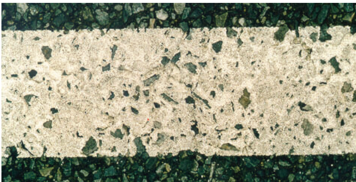
FIGURE L3 85% OF AREA INTACT
