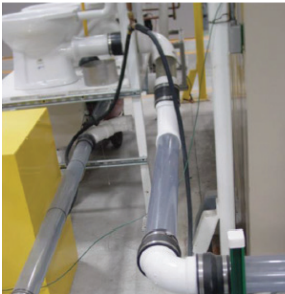
(e) Toilet with back outlet connected to a 100 mm drain line
