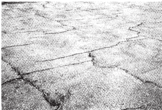
FIG. X1.17 Medium-Severity Block Cracking
