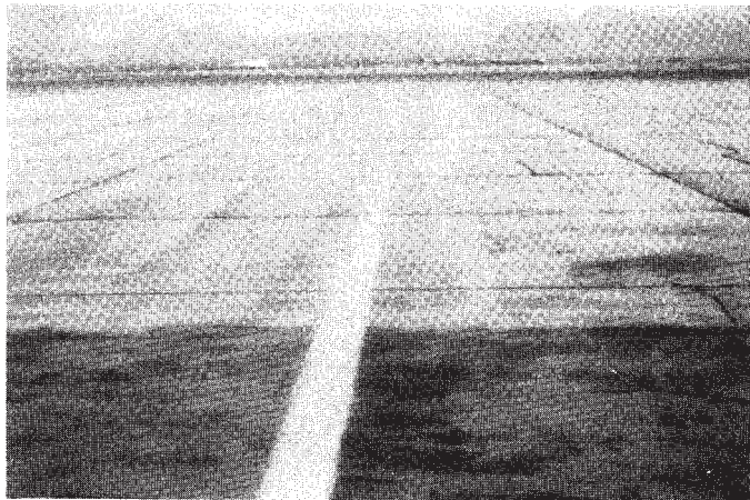
FIG. X1.30 Low-Severity Joint Reflection Cracking
