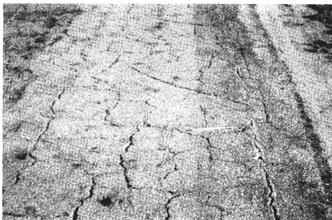
FIG. X1.20 High-Severity Block Cracking
