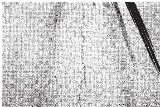
FIG. X1.32 Low-Severity Joint Reflection Cracking, Nonfilled Crack
