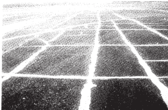
FIG. X1.13 Low-Severity Block Cracking, Filled Cracks
