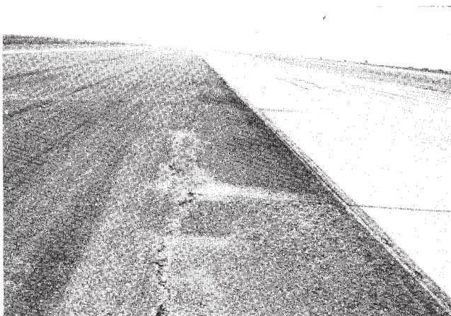
FIG. X1.41 Medium-Severity Longitudinal Crack
