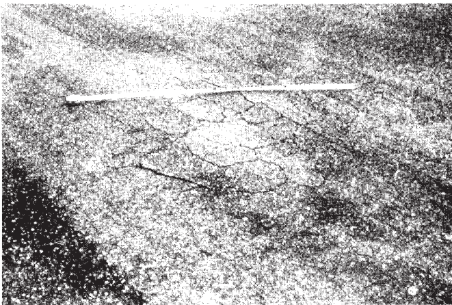
FIG. X1.7 Medium-Severity Alligator Cracking, Approaching High Severity (Example 1)
