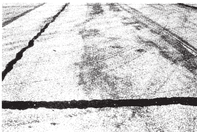
FIG. X1.31 Low-Severity Joint Reflection Cracking, Filled Crack
