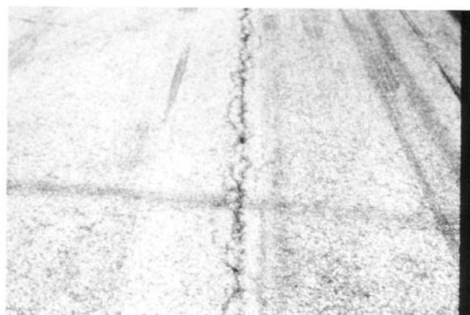
FIG. X1.39 Medium-Severity Longitudinal Construction Joint Crack
