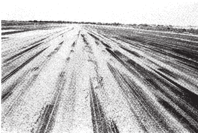
FIG. X1.38 Low-Severity Longitudinal Cracks, Approaching Medium
