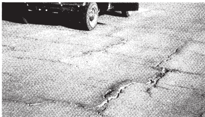
FIG. X1.18 High-Severity Block Cracking
