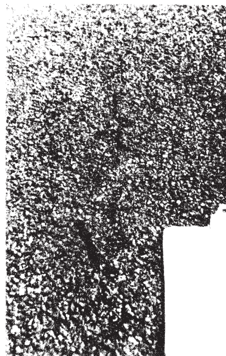
FIG. X1.44 Medium-Severity Crack in Porous Friction Course
