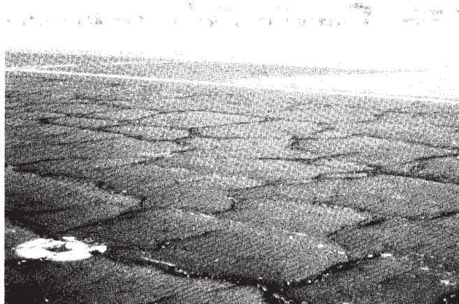
FIG. X1.19 High-Severity Block Cracking
