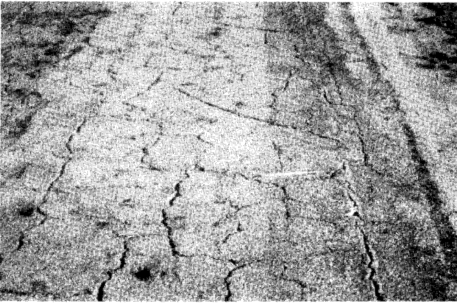
FIG. X1.20 High-Severity Block Cracking
