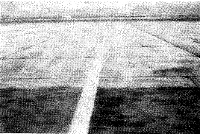
FIG. X1.30 Low-Severity Joint Reflection Cracking
