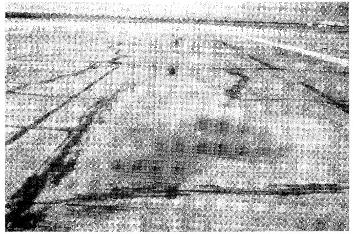
FIG. X1.27 High-Severity Depression (2 in. (50 mm))
