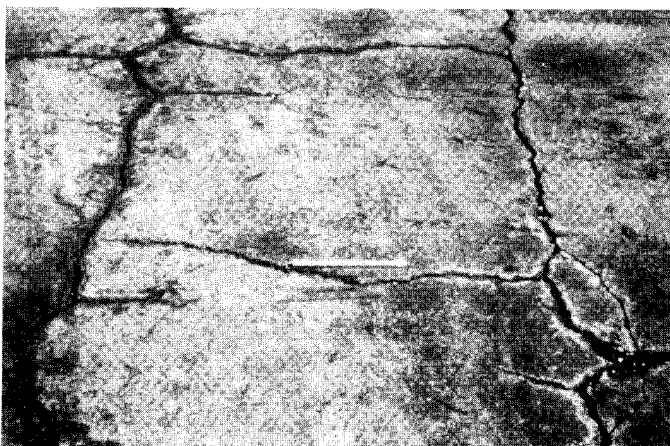
FIG. X1.16 Medium-Severity Block Cracking
