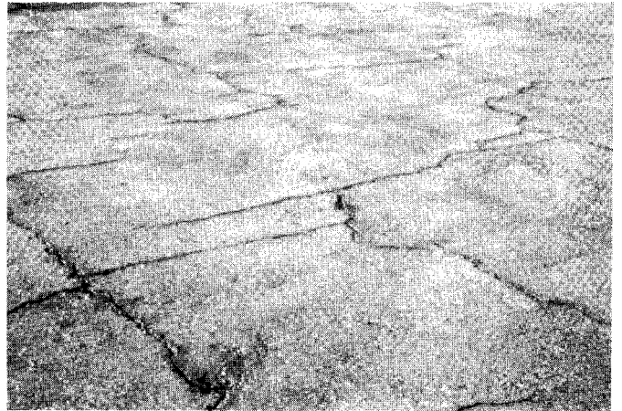
FIG. X1.17 Medium-Severity Block Cracking
