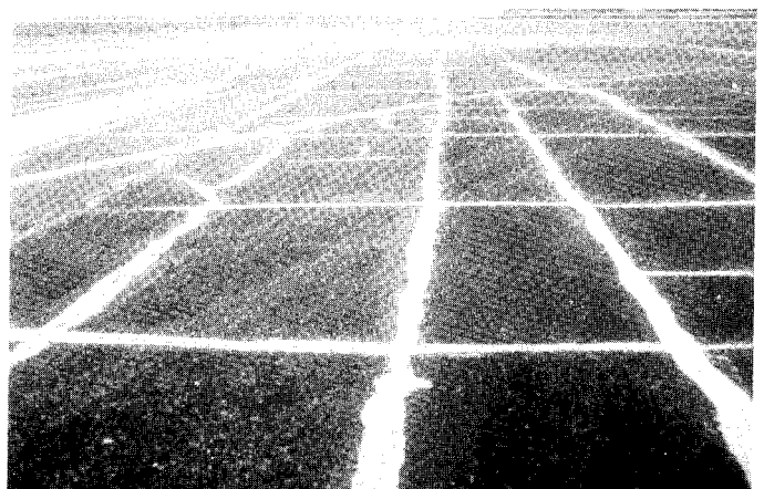
FIG. X1.13 Low-Severity Block Cracking
