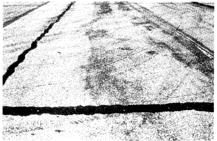
FIG. X1.31 Low-Severity Joint Reflection Cracking, Filled Crack
