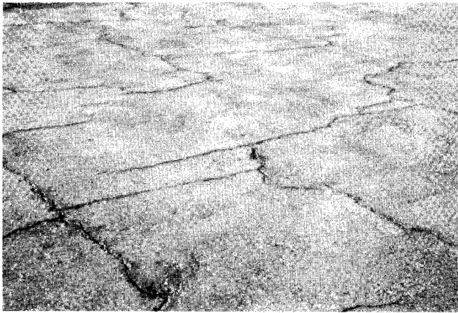
FIG. X1.17 Medium-Severity Block Cracking
