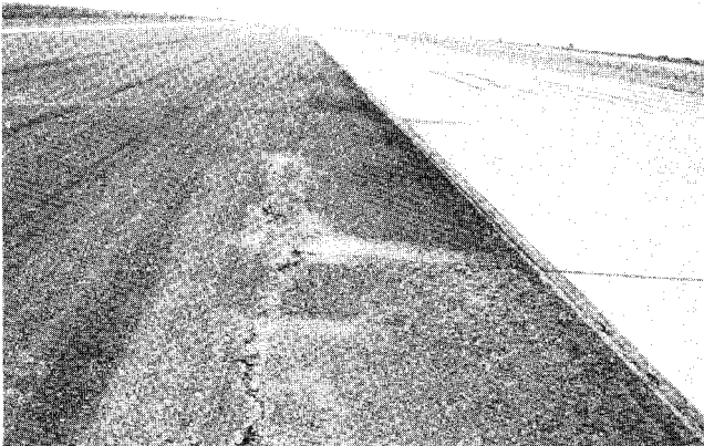
FIG. X1.41 Medium-Severity Longitudinal Crack
