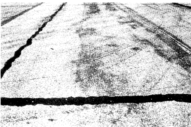
FIG. X1.31 Low-Severity Joint Reflection Cracking, Filled Crack
