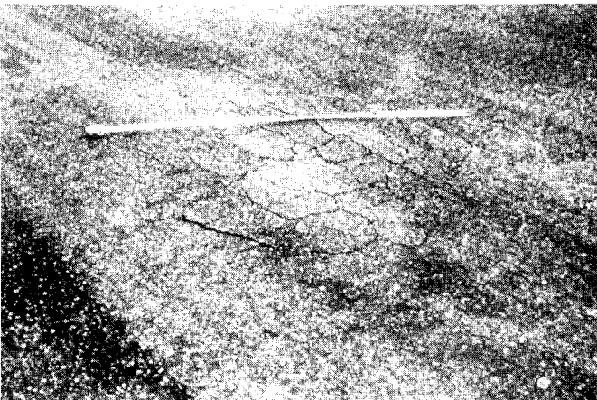
FIG. X1.7 Medium-Severity Alligator Cracking, Approaching High Severity (Example 1)
