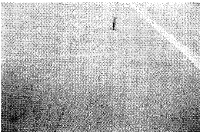
FIG. X1.1 Low-Severity Alligator Cracking
