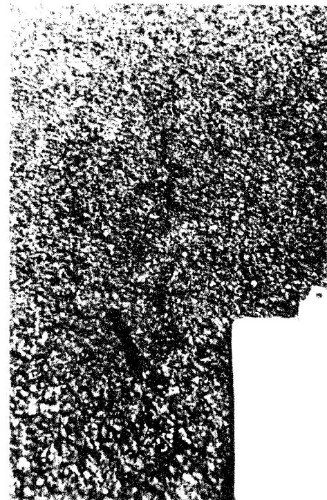
FIG. X1.44 Medium-Severity Crack in Porous Friction Course
