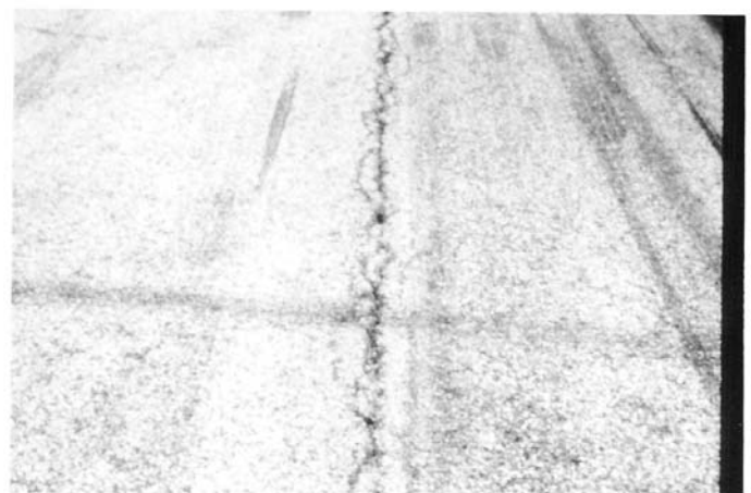
FIG. X1.39 Medium-Severity Longitudinal Construction Joint Crack
