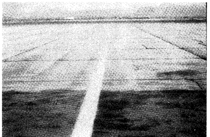
FIG. X1.30 Low-Severity Joint Reflection Cracking
