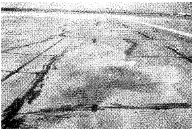
FIG. X1.27 High-Severity Depression (2 in. (50 mm))
