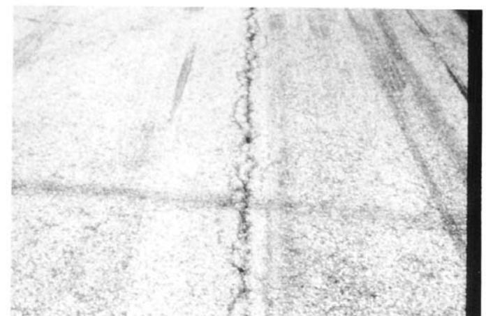
FIG. X1.39 Medium-Severity Longitudinal Construction Joint Crack
