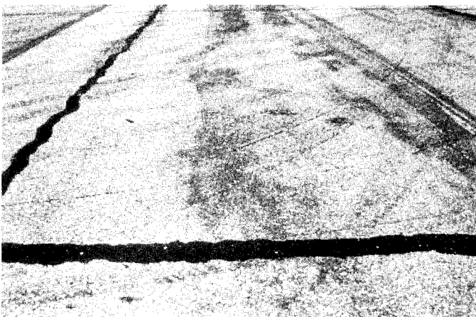
FIG. X1.31 Low-Severity Joint Reflection Cracking, Filled Crack
