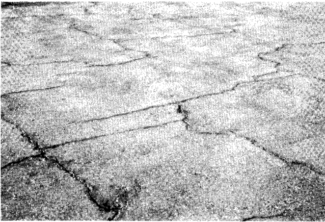
FIG. X1.17 Medium-Severity Block Cracking
