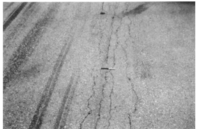
FIG. X1.3 Low-Severity Alligator Cracking, Approaching Medium Severity
