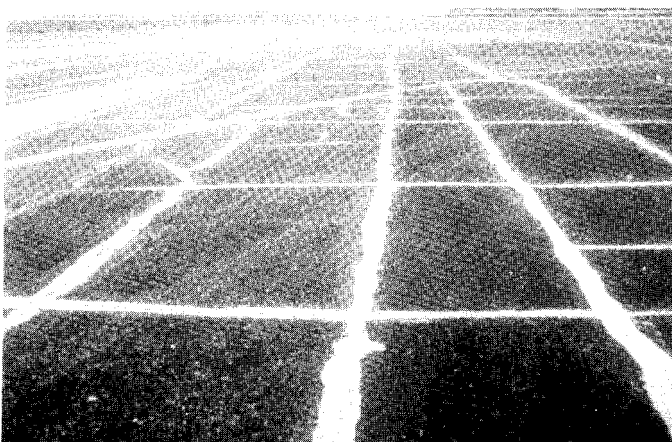
FIG. X1.13 Low-Severity Block Cracking, Filled Cracks
