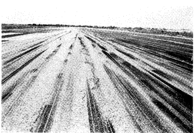
FIG. X1.38 Low-Severity Longitudinal Cracks, Approaching Medium
