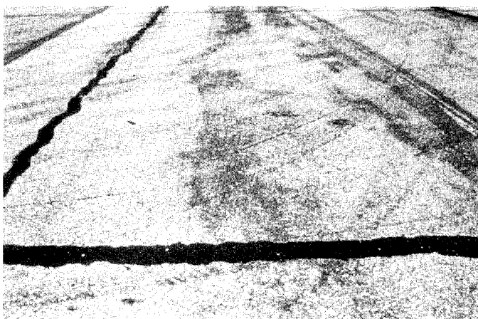
FIG. X1.31 Low-Severity Joint Reflection Cracking, Filled Crack
