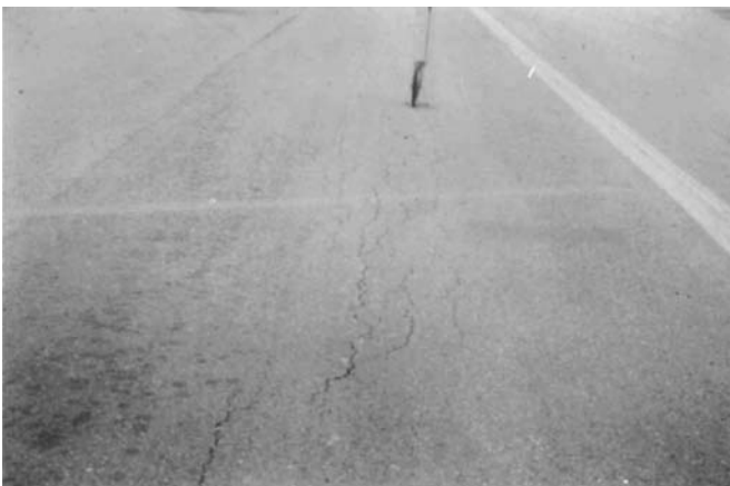
FIG. X1.1 Low-Severity Alligator Cracking
