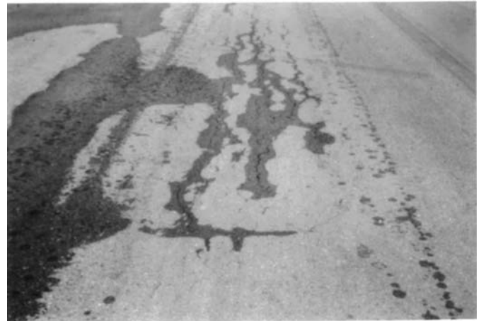
FIG. X1.2 Low-Severity Alligator Cracking
