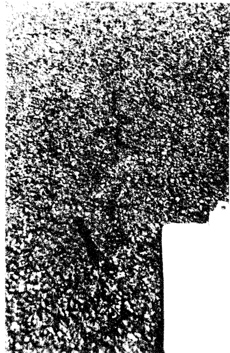
FIG. X1.44 Medium-Severity Crack in Porous Friction Course
