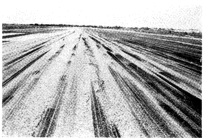
FIG. X1.38 Low-Severity Longitudinal Cracks, Approaching Medium
