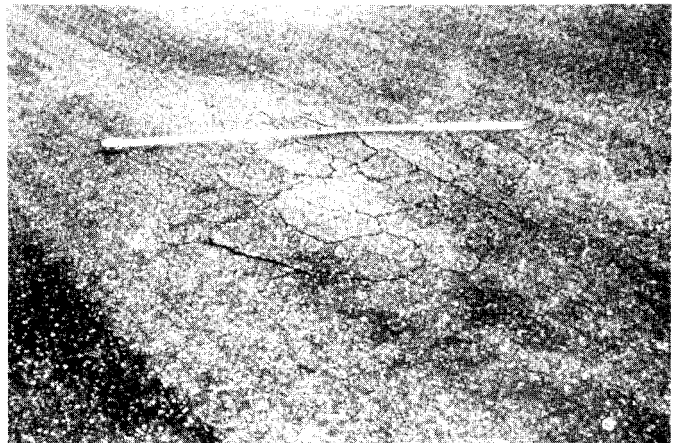
FIG. X1.7 Medium-Severity Alligator Cracking, Approaching High Severity (Example 1)
