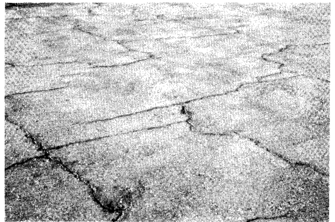
FIG. X1.17 Medium-Severity Block Cracking
