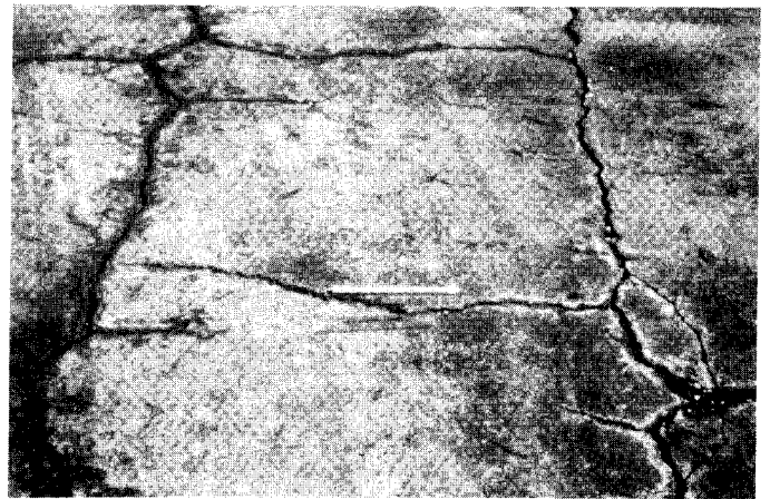
FIG. X1.16 Medium-Severity Block Cracking
