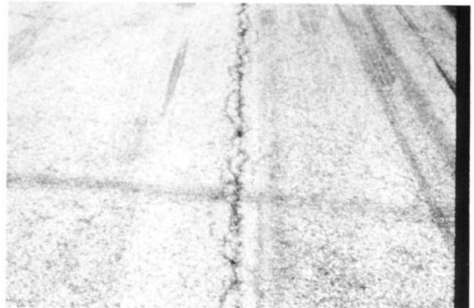
FIG. X1.39 Medium-Severity Longitudinal Construction Joint Crack
