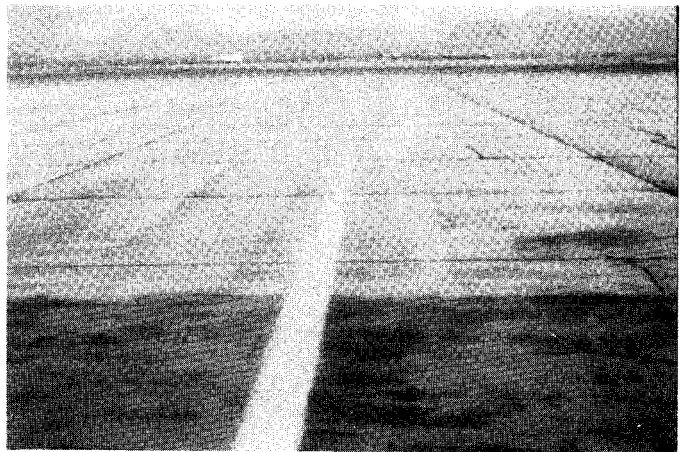
FIG. X1.30 Low-Severity Joint Reflection Cracking
