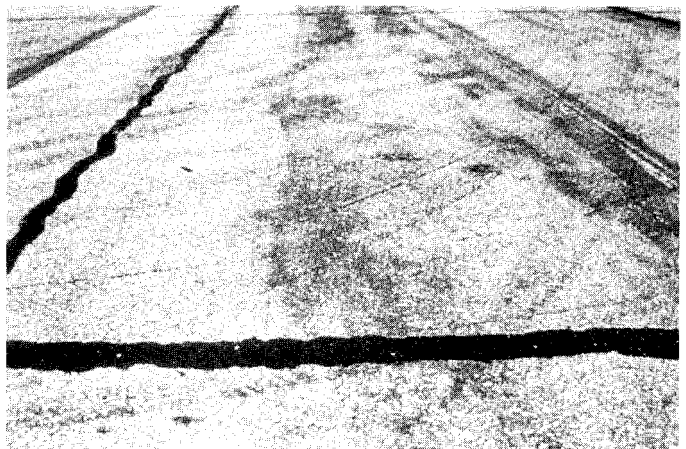
FIG. X1.31 Low-Severity Joint Reflection Cracking, Filled Crack
