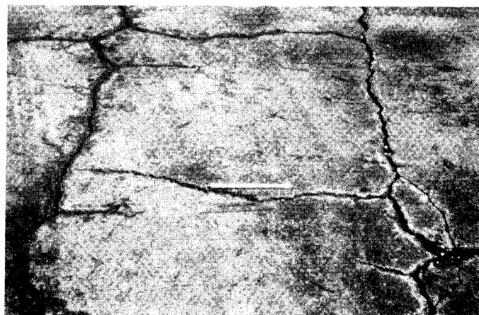
FIG. X1.16 Medium-Severity Block Cracking
