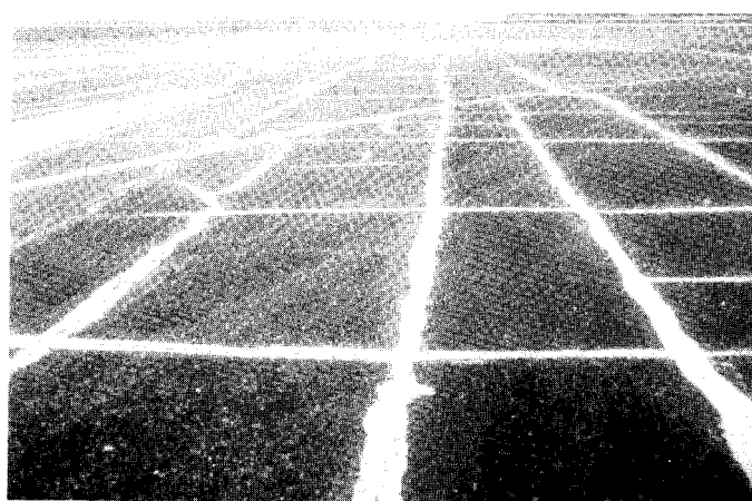
FIG. X1.13 Low-Severity Block Cracking, Deep Cracks
