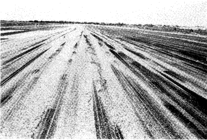
FIG. X1.38 Low-Severity Longitudinal Cracks, Approaching Medium
