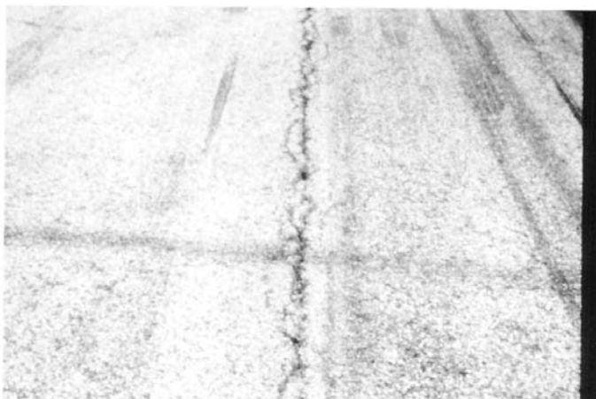
FIG. X1.39 Medium-Severity Longitudinal Construction Joint Crack
