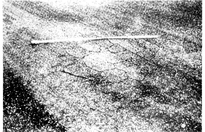
FIG. X1.7 Medium-Severity Alligator Cracking, Approaching High Severity (Example 1)
