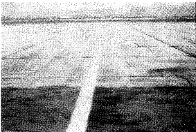
FIG. X1.30 Low-Severity Joint Reflection Cracking
