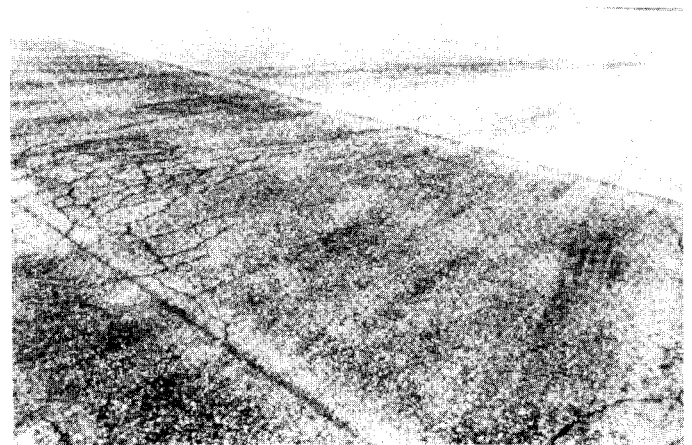
FIG. X1.8 Medium-Severity Alligator Cracking, Approaching High Severity (Example 2)
