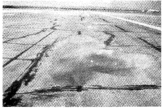
FIG. X1.27 High-Severity Depression (2 in. (50 mm))
