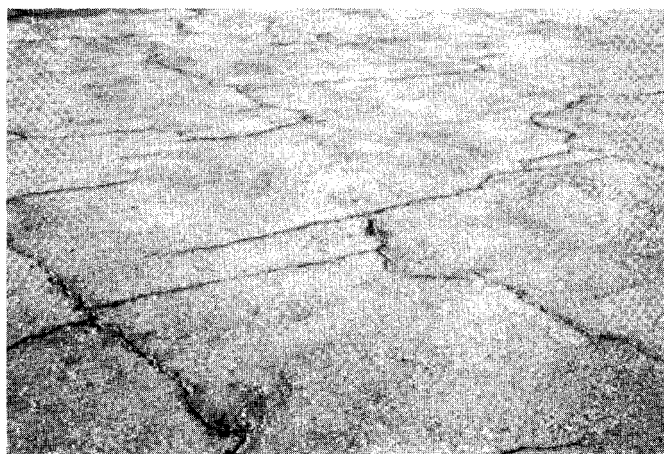
FIG. X1.17 Medium-Severity Block Cracking
