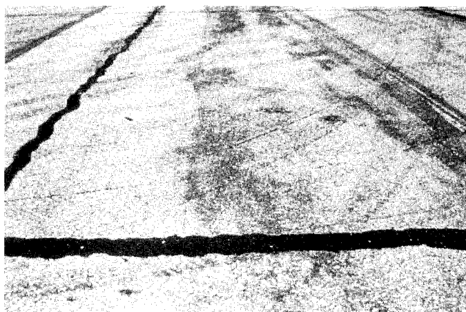
FIG. X1.31 Low-Severity Joint Reflection
