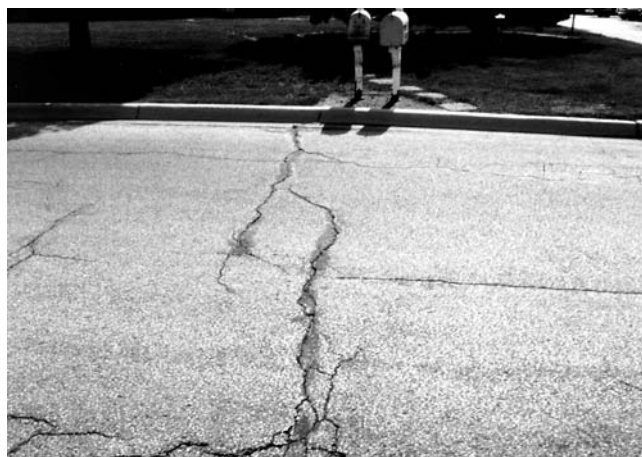
FIG. X1.8 Medium-Severity Block Cracking
