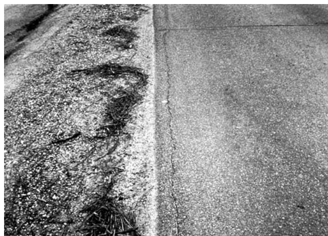
FIG. X1.19 Low-Severity Edge Cracking
