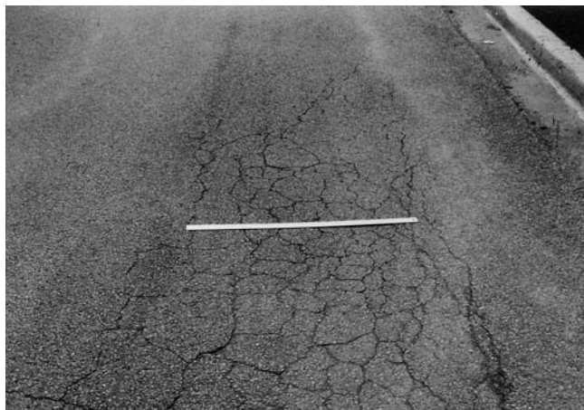
FIG. X1.2 Medium-Severity Alligator Cracking
