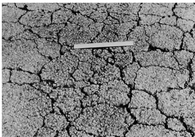
FIG. X1.3 High-Severity Alligator Cracking
