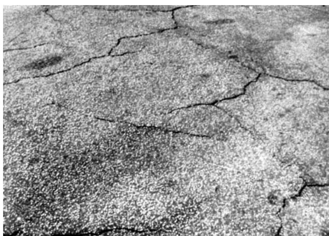
FIG. X1.9 High-Severity Block Cracking
