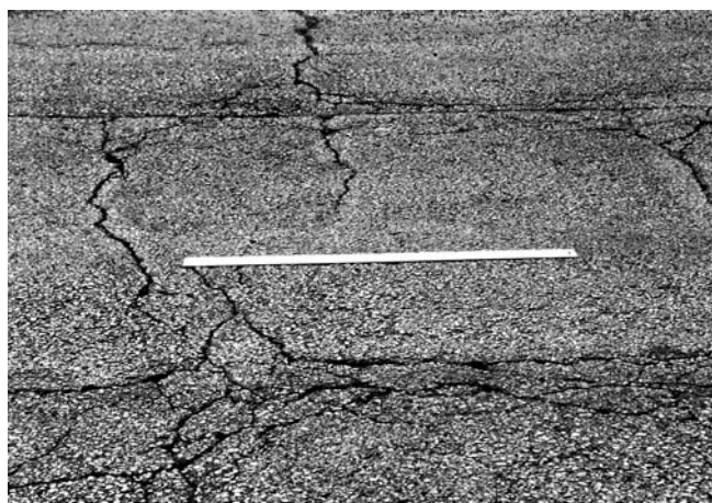
FIG. X1.7 Low-Severity Block Cracking
