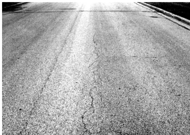
FIG. X1.1 Low-Severity Alligator Cracking
