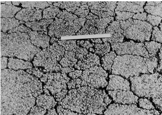
FIG. X1.3 High-Severity Alligator Cracking
