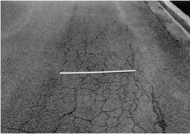
FIG. X1.2 Medium-Severity Alligator Cracking
