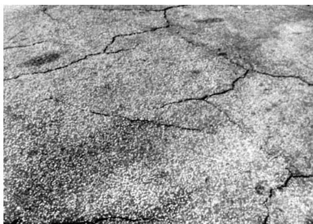
FIG. X1.9 High-Severity Block Cracking
