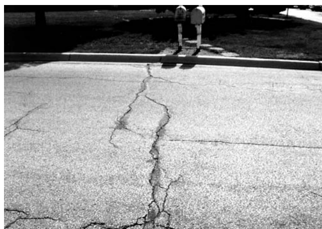
FIG. X1.8 Medium-Severity Block Cracking
