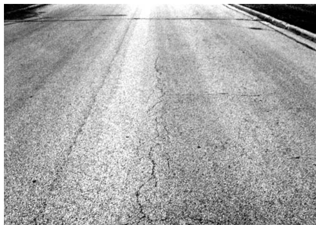
FIG. X1.1 Low-Severity Alligator Cracking
