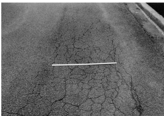
FIG. X1.2 Medium-Severity Alligator Cracking
